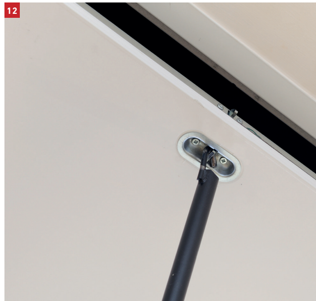
Using the operating pole for opening the drop-down door
